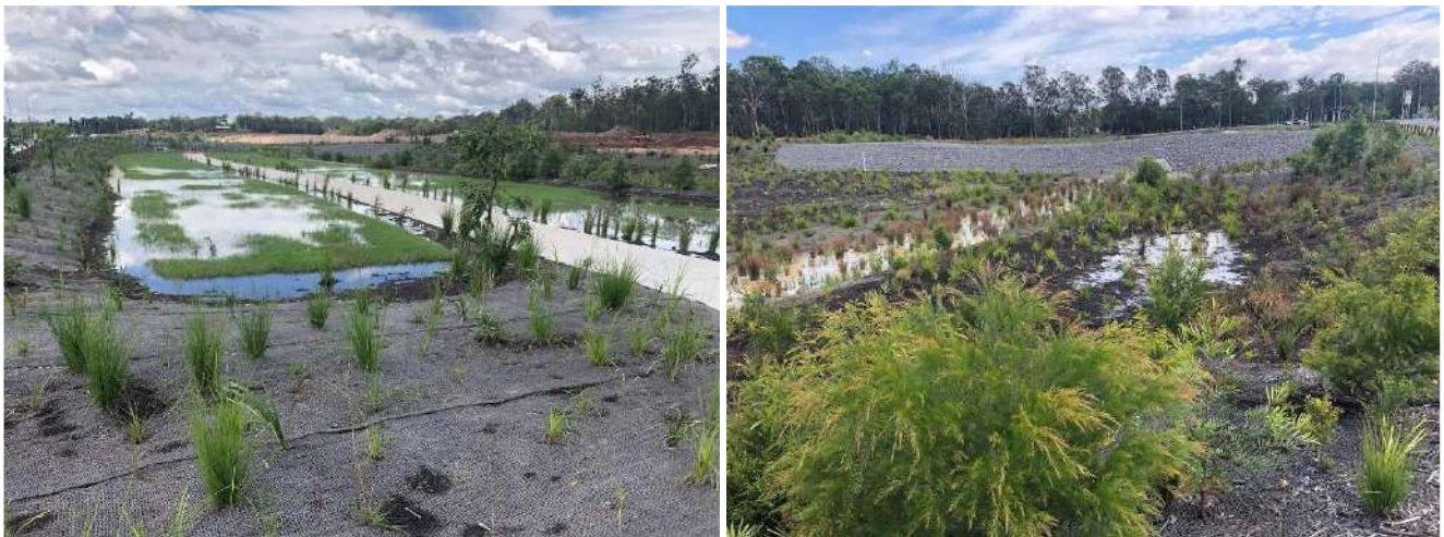
Photo Set 1: Construction and planting of northern Stage 1 basin and rehabilitation of waterway.
