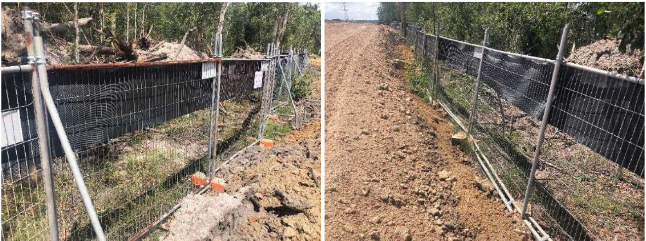
Photo Set 4: Temporary koala exclusion fencing installed along some of the construction area boundaries.
